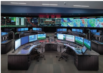
Cal ISO Headquarters Data Center, Folsom
