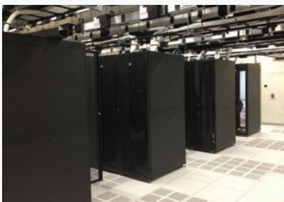
Modesto Junior College Tech Center New Data Center, Modesto
